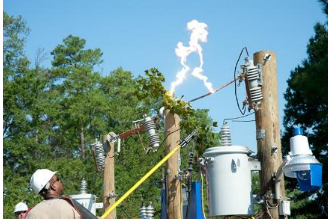
Figure 1.4 – Example of an arc caused by a tree limb (Photo by the Knoxville Utilities Board)
